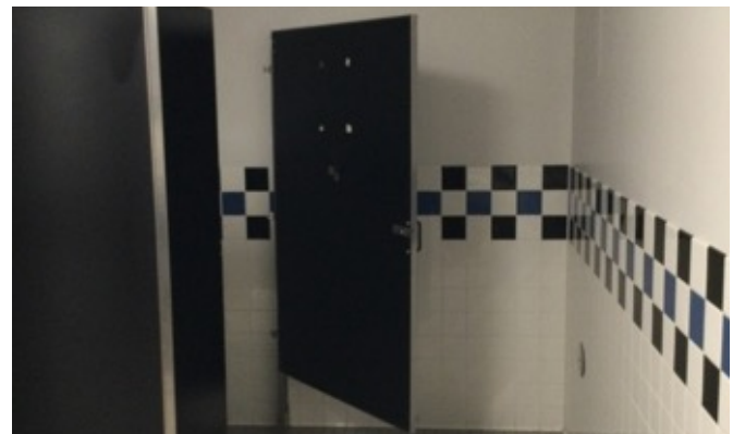
Non-compliant Restroom Door Entrances and Outdated Restroom Finishes
