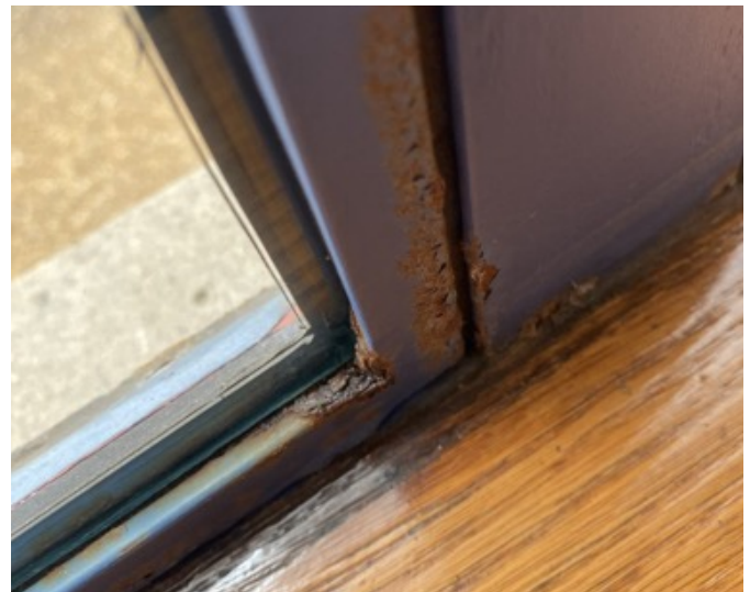
Rust on the bottom sill of windows from condensation
