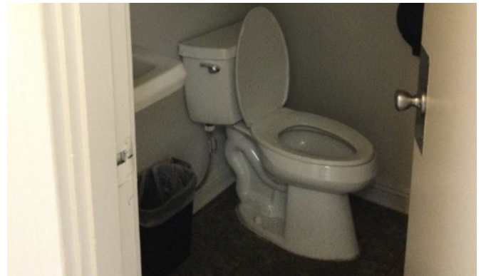
The single Library restroom does not have proper floor clearances.
